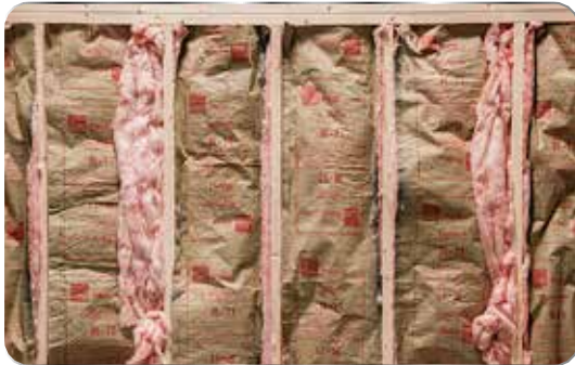
R-13 Batten Insulation In Walls & Ceiling
